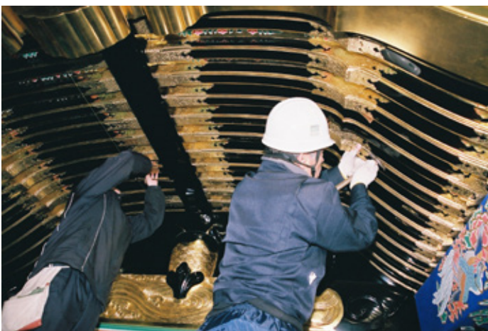
Craftsmen attach repaired metal fittings to the Yomeimon Gate Photo: Courtesy of Association for the Preservation of the Nikko World Heritage Site Shrines and Temples
