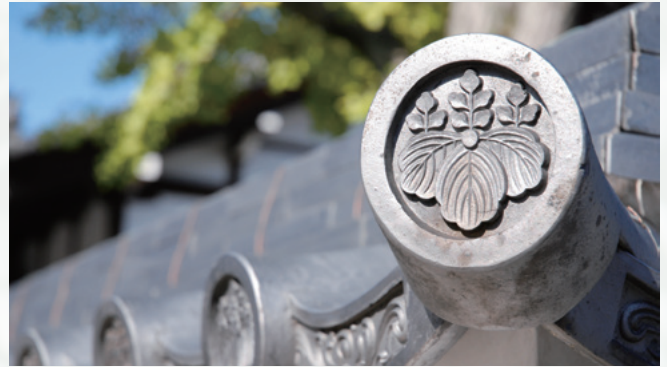
Kamon crests can also be seen adorning yane-gawara roof tiles used in Japanese structures, including castles, temples, shrines, and houses built with traditional techniques. Shown in the photo is a kiri-mon 4 crest.
